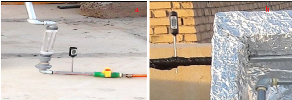
Fig. 2. (a) Pipe at inlet and (b) pipe at outlet.
