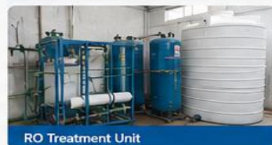
RO Treatment Unit
