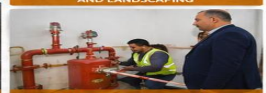
SAFETY AND FIRE SYSTEMS
