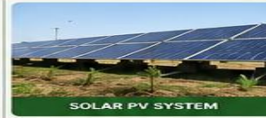
SOLAR PV SYSTEM
