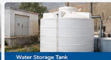
Water Storage Tank
